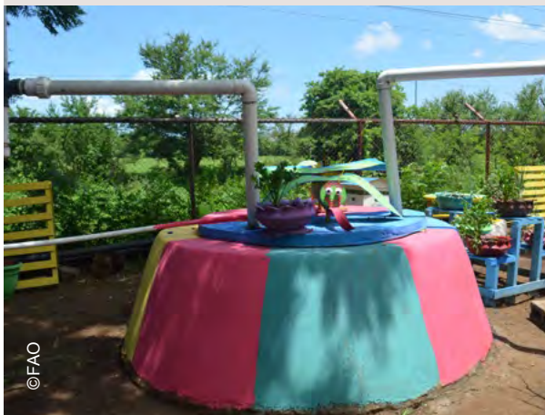
Managua, Nicaragua. Tank to store rainwater, installed by the municipality
